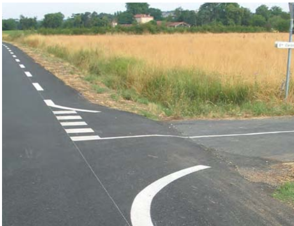
The marking abruptly interrupts the cyclist's path
