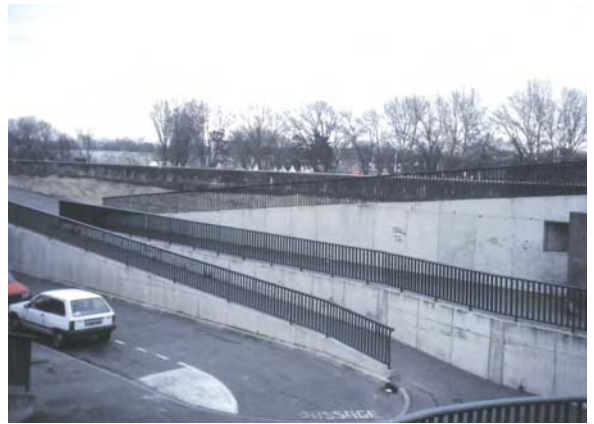
The bridge is accessible to persons with reduced mobility by a ramp with landings (ST Toulouse)
