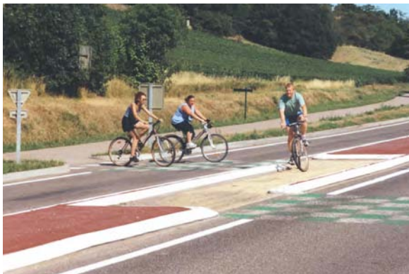
Staggered barriers slow down cyclists but limit the number who can queue (Certu)
