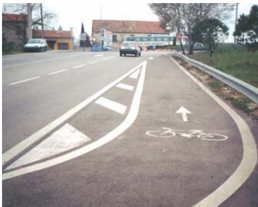
Separation can be made depending on the case, by a refuge island or a hatched area (Certu)
