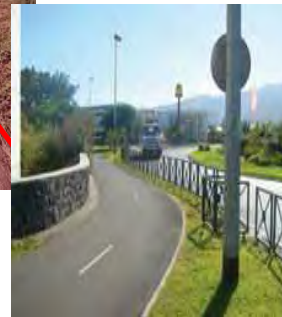
A path with good maintenance is a path able to be used by cyclists
