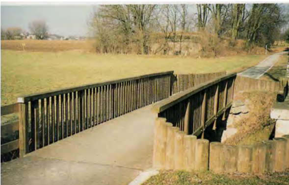
1.4 m safety grille for cyclists
